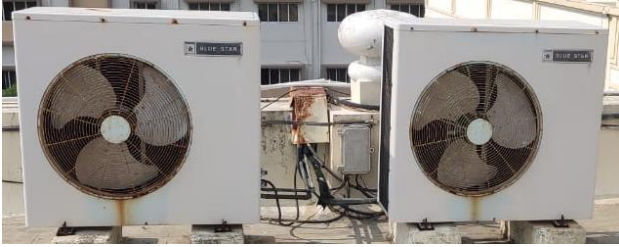
Conference hall outdoor unit – 11 TR (4 nos.)
