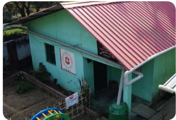
Rainwater Harvesting Structure
