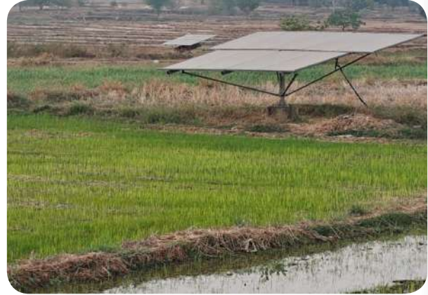
Solar-powered irrigation pumps
