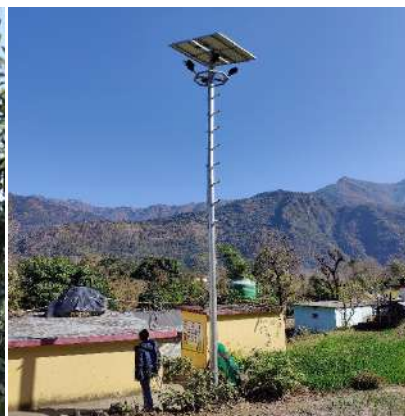
FIGURE 8: SOLAR STREET LIGHTS
