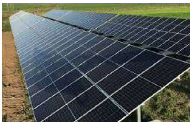
FIGURE 1.7: SOLAR PANELS AT PALLI GP, JAMMU
