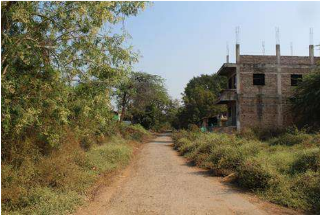
Image 7.3: Concrete Road Washed away because of Rain (Source- Author)
