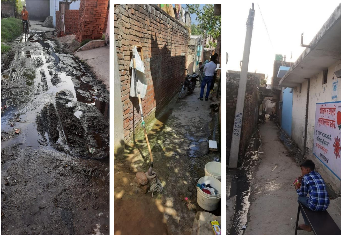
Figure 38 a) Wastewater overflow on road, b) Lack of proper drains, c) uncovered drains
