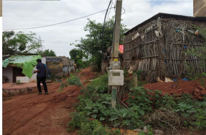
Typical kuchha road with damages
