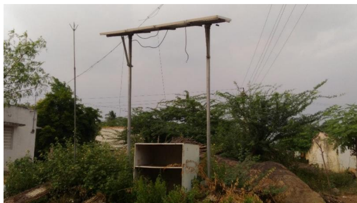
Figure 6.10: Solar Panels for streetlighting
