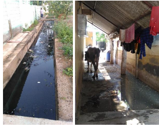
Figure 6.7d: Water stagnation in house
