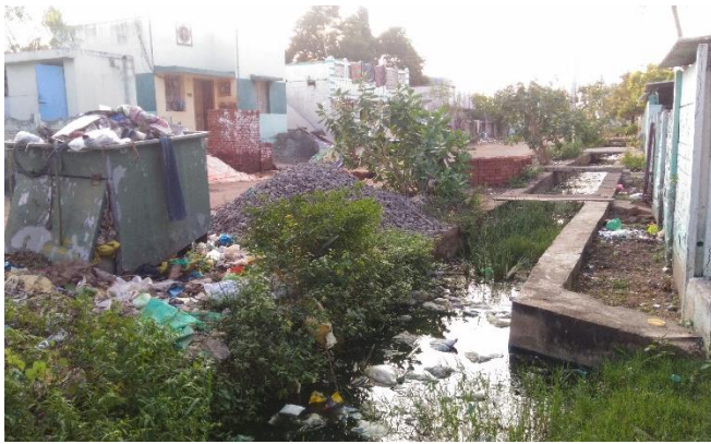
Figure 6.7c: Poorly maintained drains
