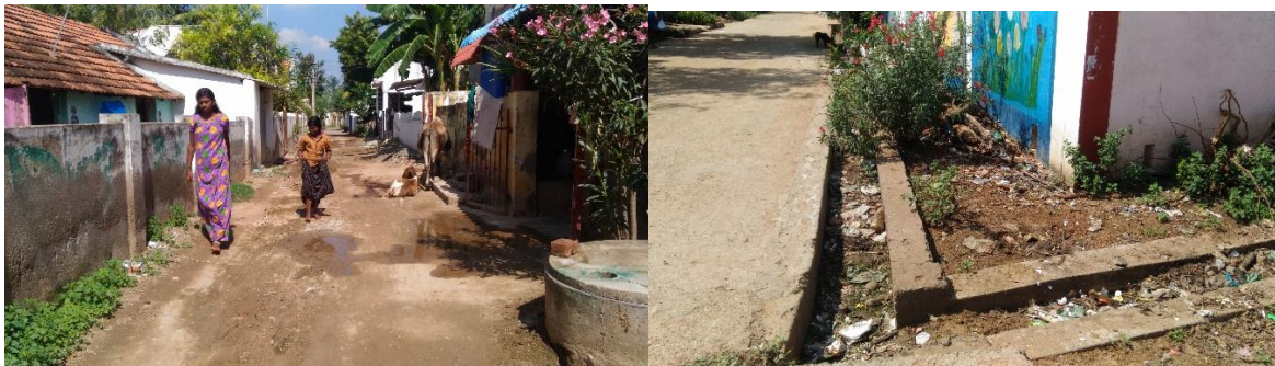
Figure 6.7f: Street stagnated with grey water Figure 6.7g: Closed drains
