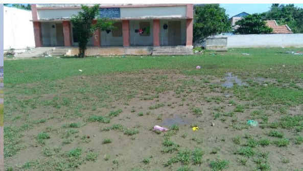
Figure 6.7b: Water stagnation in ground
