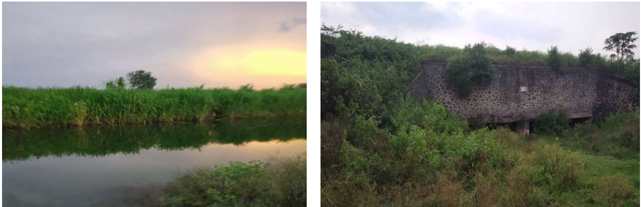
Figure 3:14. Canal along the farmland and dilapidated walls of canal over a stream culvert
