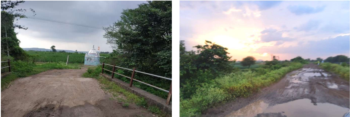
Figure 2.8 Culverts on Kukadi Canal without safety barriers
