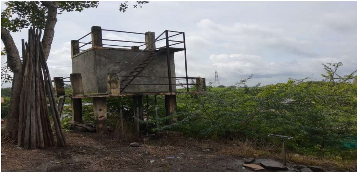
Figure 2:7. Elevated Water Storage
