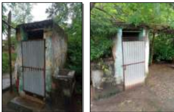
Fig. 6.6: Toilets built under Swachh Bharat Mission Source: Author
