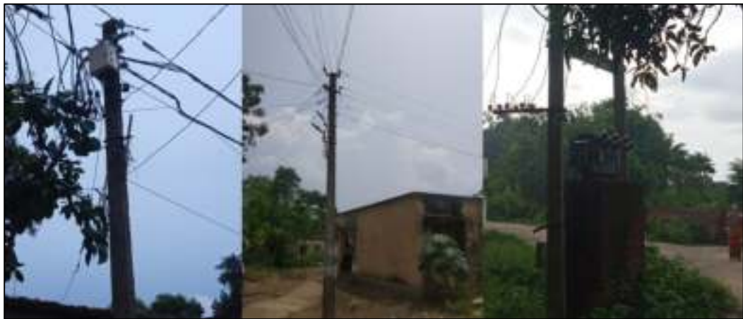
Fig. 6.15: Existing Condition of the lighting system in Kandra GP
