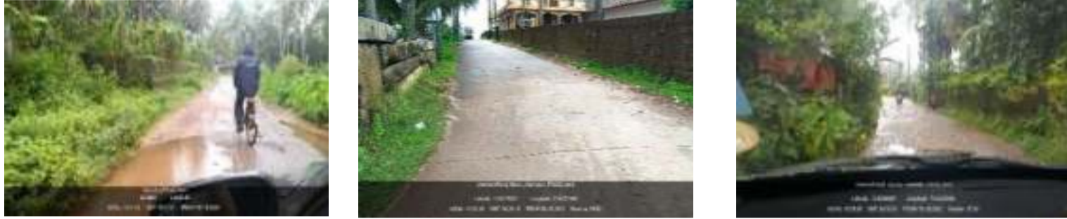
Figure 8-7 Road Network (a).Approach Road towards NH66, (b).Concrete Road, Bijoor, (c).Concrete Road, Bijoor (MSAP, 2020)
