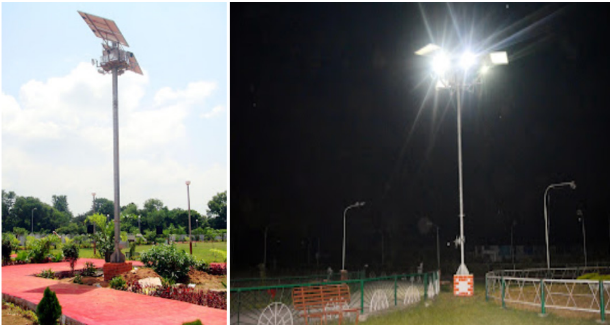
Solar powered High Mast LED light installed in Raipur, Chhattisgarh
