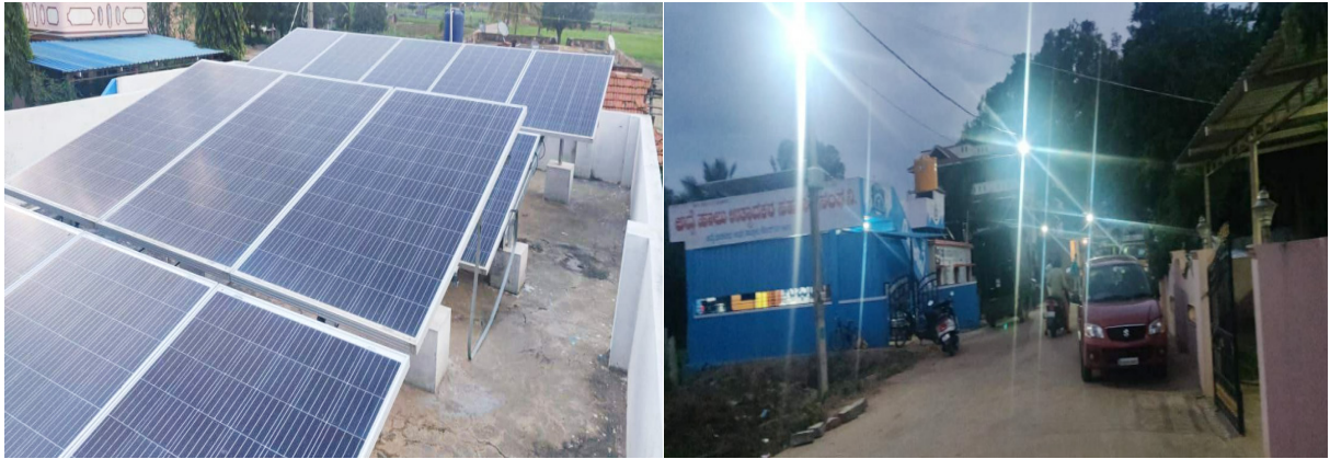
Solar Rooftop model adopted by Rajanukunte Village in Karnataka for Streetlighting using XV FC funds
