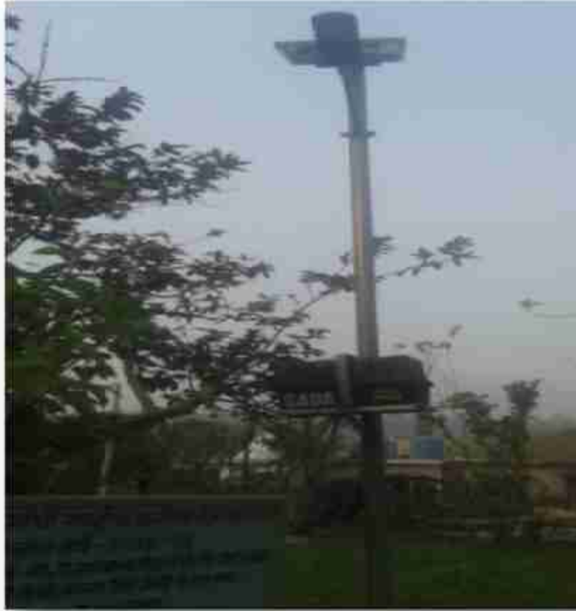
Image: Street Light installed in the GP
