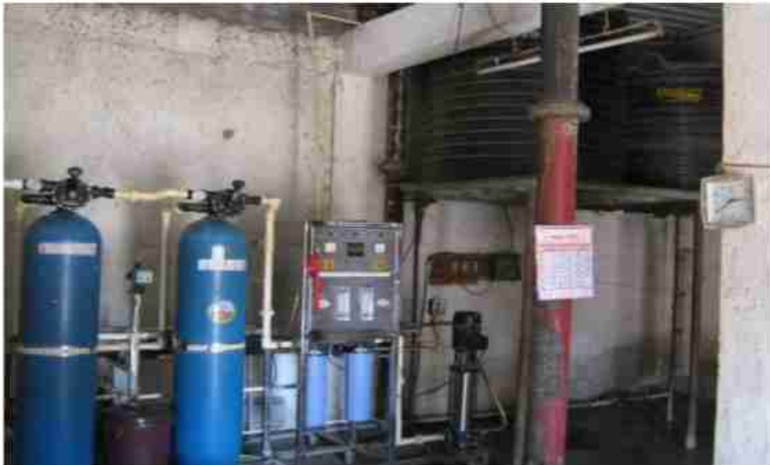
Reverse Osmosis Water Purifying Plant, Karcheliya Gram Panchayat
