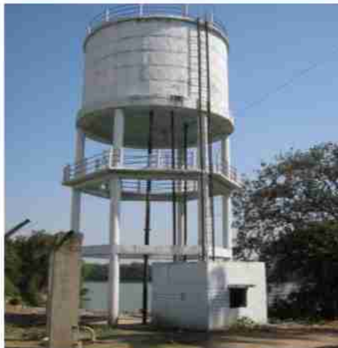
Water Tank, Ras Gram Panchayat
