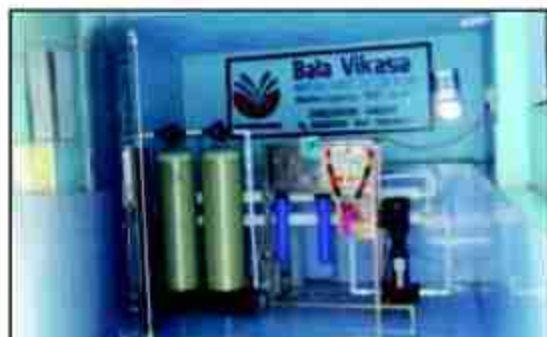
Water Treatment Plant, Shelgaon Gauri GP
