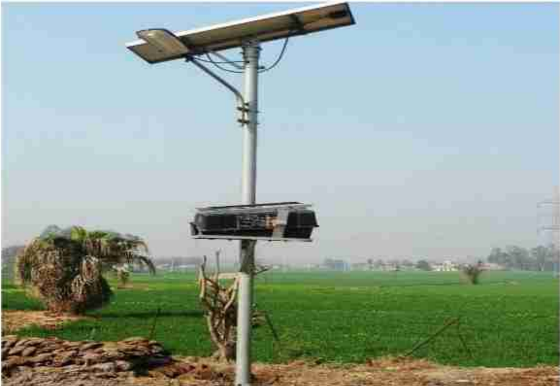
Solar Powered Lights in Harnampura Gram Panchayat
