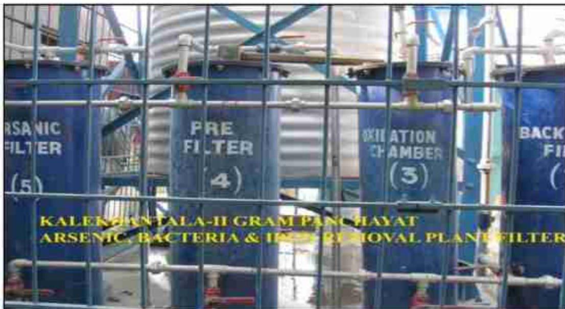
Kalekhantala - II Gram Panchayat Arsenic, Bacteria & Iron Removal Plant Filter
