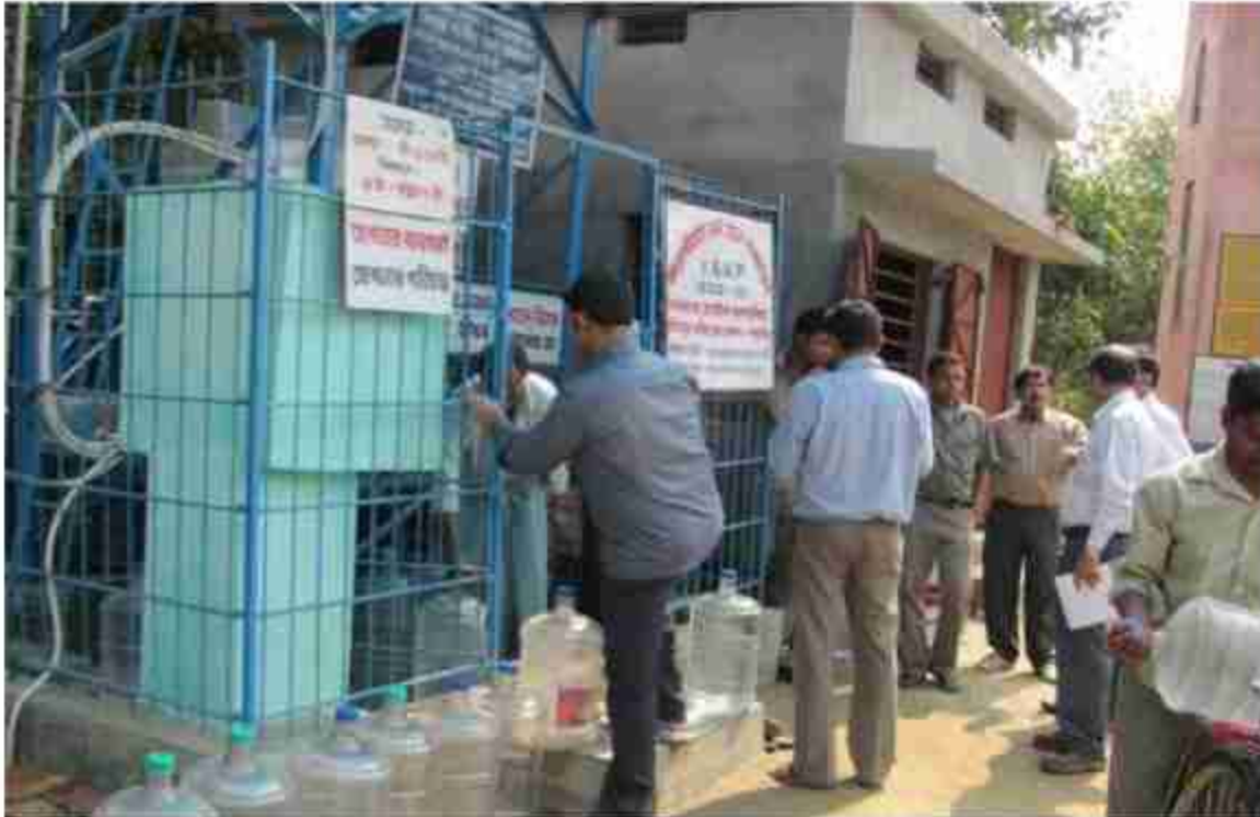
Kalekhantala – II Gram Panchayat Water Treatment Plant
