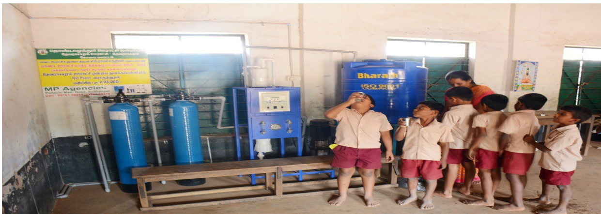
Picture of Reverse Osmosis Plant in a School
