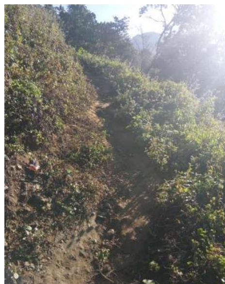
Porter track constructed under BRGF from Hill top to colony Taliha to Dupit,Eba-I GP,Taliha Block,Upper Subansiri District, Arunachal Pradesh
