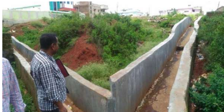
Construction of CC drain from Gandhinagar Samsan towards Astaprahare Sunabeda Municipality, Koraput District, Odisha State
