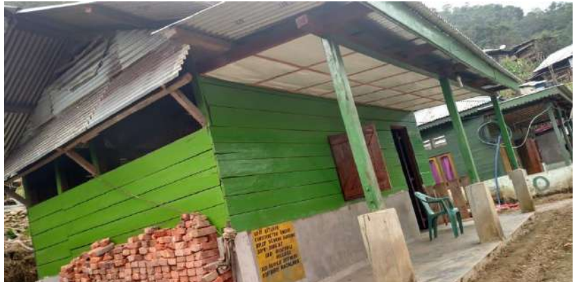
Construction of Kitchen for VDB under BRGF in Old Risethsi Village, Kiphire District, Nagaland State
