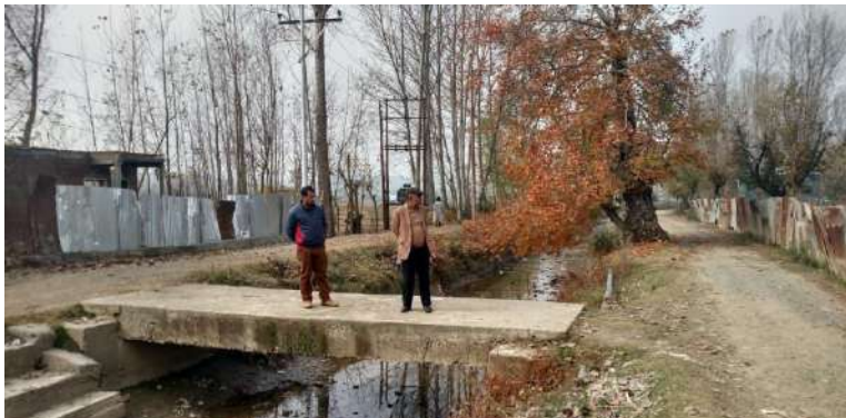
Construction of Culvert under BRGF in Tangdar A GP, Kupwara District, Jammu & Kashmir State
