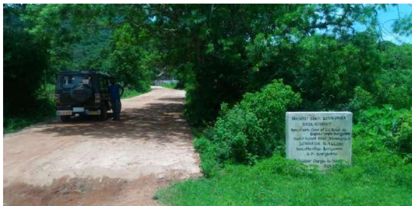
Construction of CC road under BRGF in Borigumma GP, Koraput District, Odisha State
