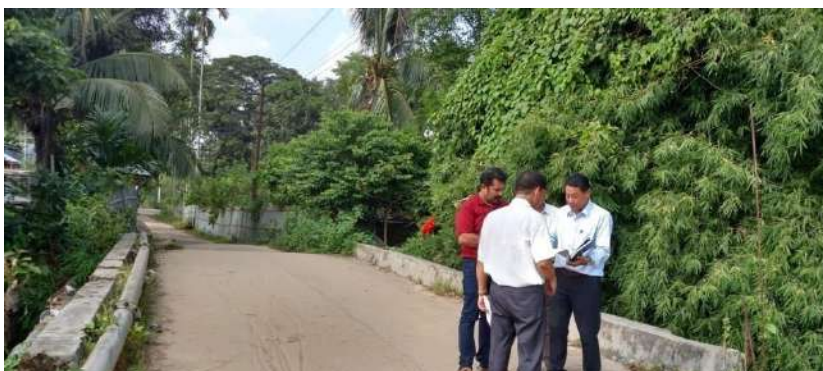
Formation of Road under BRGF from Biswaram Para to Dabaram Para, Dhalai District, Tripura State
