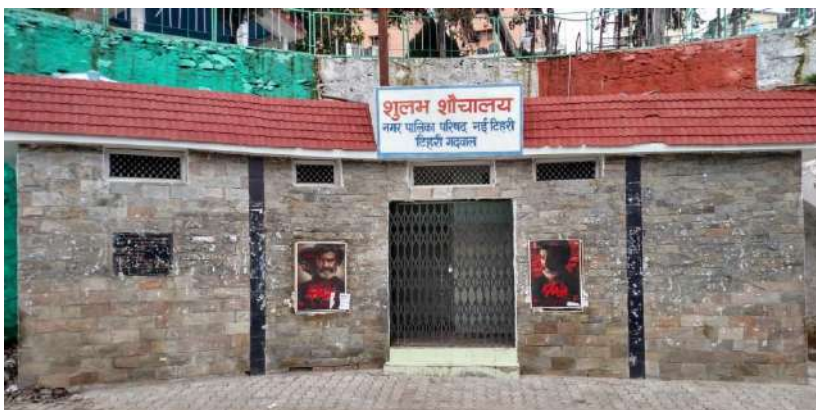
Construction of Toilet Complex under BRGF in New Thehari Municipality, Tehri Garhwal District, Uttarakhand State
