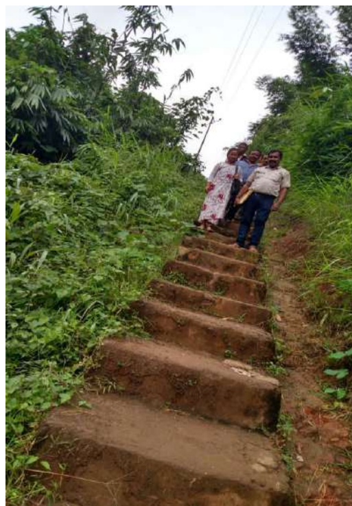
Construction of Steps under BRGF in Lungpher GP, Sangau Block, Lawntlai District, Mizoram State
