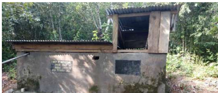
Construction of Water tank under BRGF in Tethuyo Village, Kiphire District, Nagaland State
