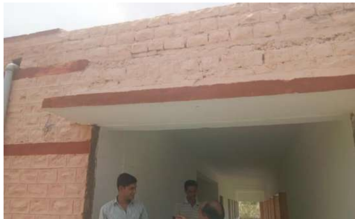
Hostel for SC Students constructed under BRGF in Jaisindhar Station GP, Gadrarod Block, Barmer District, Rajasthan State
