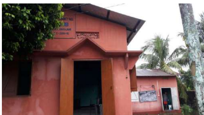
Community Hall Constructed under BRGF at Tinali Chariali GP, Kokrajar Block, Kokrajar district, Assam
