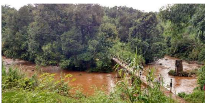
Construction of Foot Bridge over River Umran Connecting Mawlong to Qusnina under BRGF in Ri-Bhoi District, Meghalaya State
