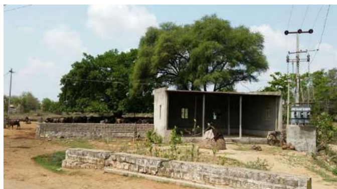
Construction of 11 KV line under BRGF Titaguri VCDC, Kokrajar Block, Kokrajar District, Assam State
