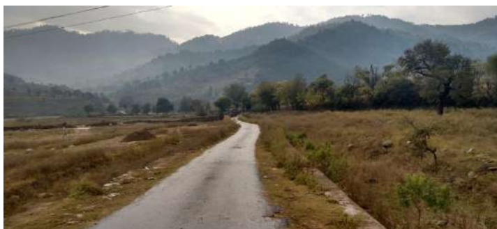
Construction of road under BRGF in Chajjala Upper GP, Poonch District, Jammu & Kashmir State
